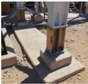
Column extensions required to lift an existing structure. Extensions designed and fabricated on site.
